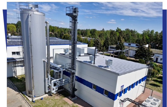
Photo: The combined heat and power unit at the Węgrów plant
