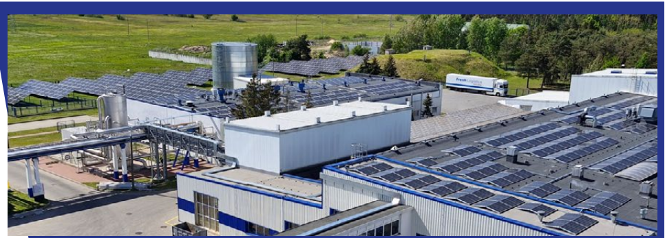
Photo: The photovoltaic system at the Węgrów plant
